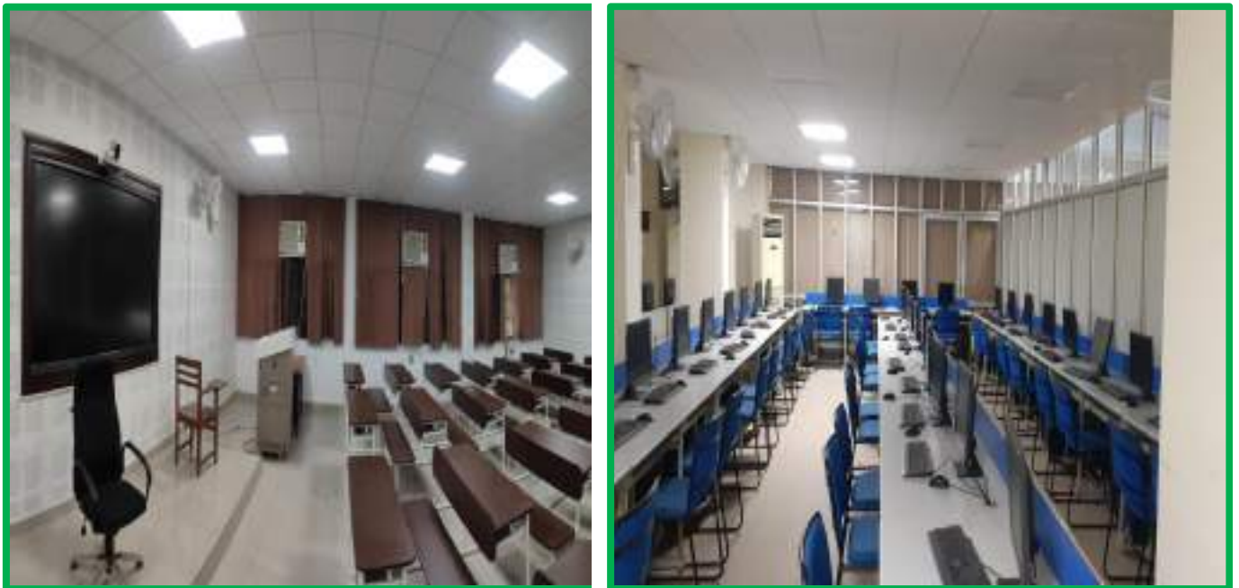
FIG 33 LED FIXTURES IN SMART CLASSROOMS (SCIENCE HALL 4, TF)
