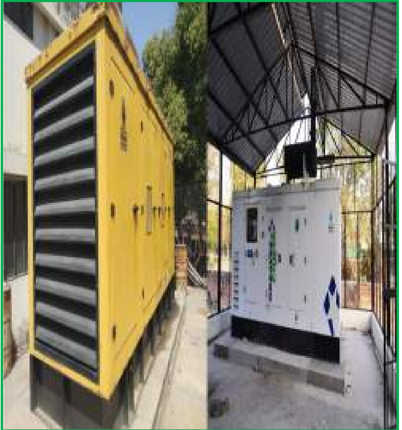
FIG. 40 DG SET INSTALLED IN ELECTRICAL WING AND ESTATE OFFICE
