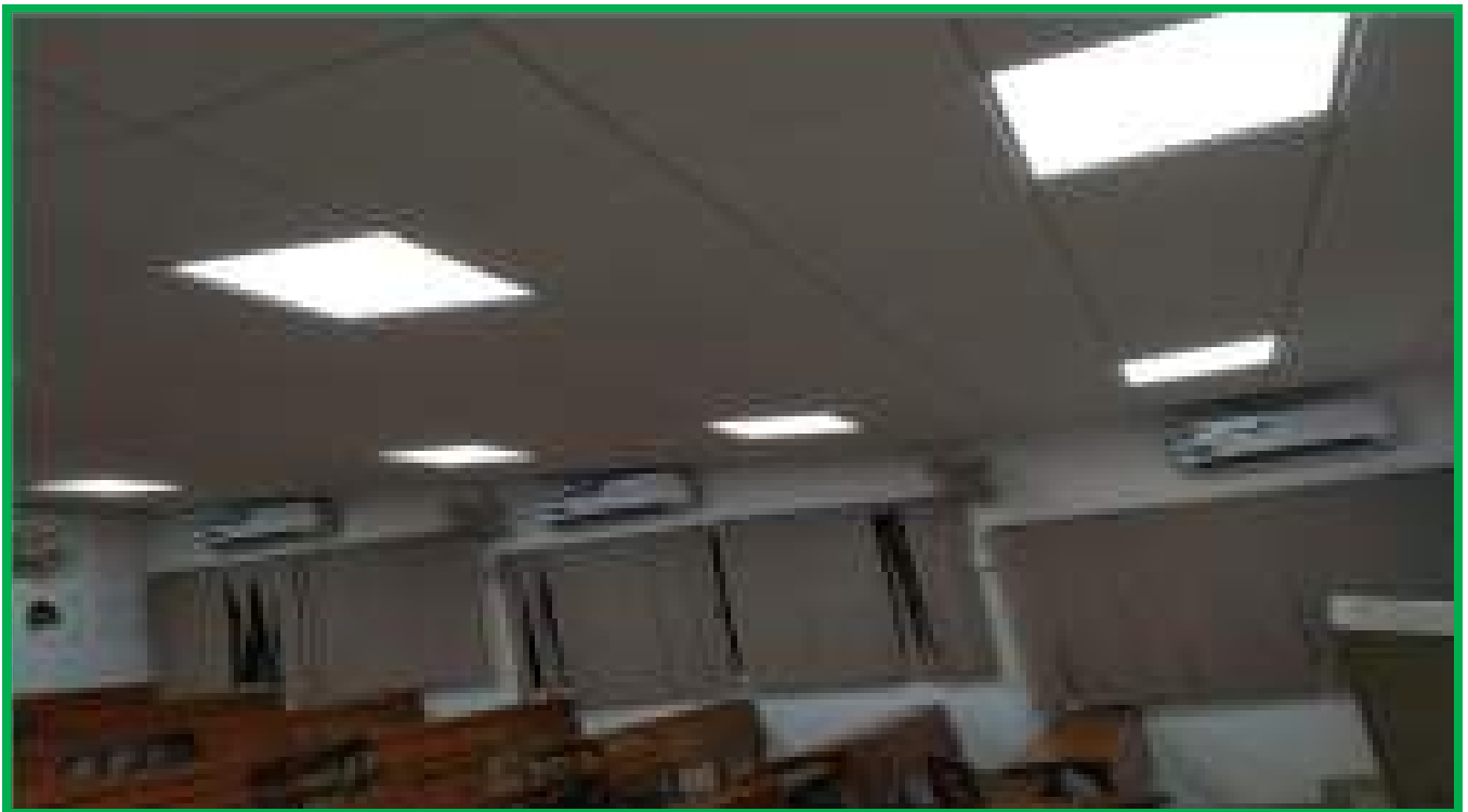
FIG. 38: STAR RATED AIR CONDITIONING IN SMART CLASSROOMS (FOOD BLOCK, LCF-I)
