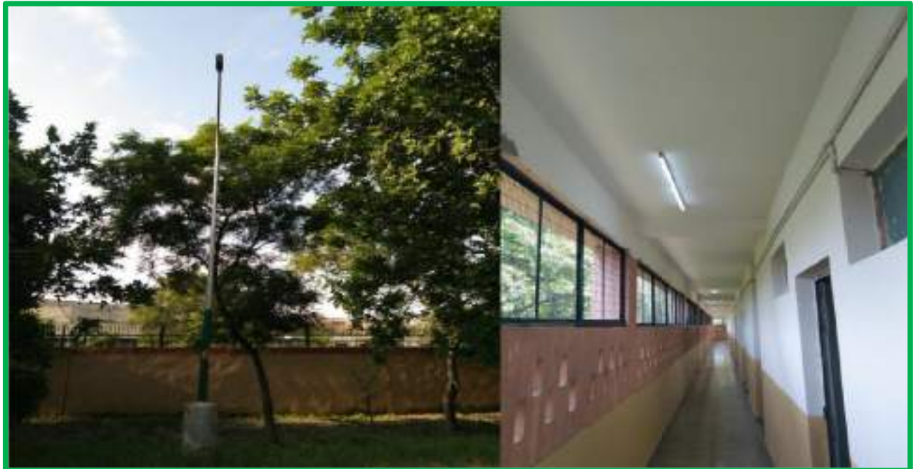
FIG 30 LED FIXTURE (STREET LIGHT, ROAD-A NEAR H POLE)/ LED FIXTURE IN GIRLS HOSTELNO.1, FF (CORRIDOR) NEAR ROOM NO. 231
