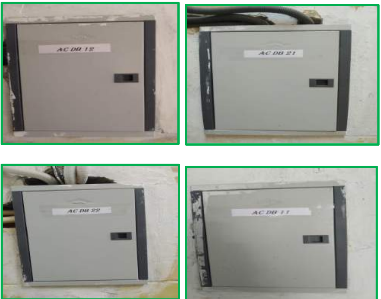
FIG 41 AC DB ATTACHED IN MECHANICAL BLOCK FOR ESSENTIAL AND NON-ESSENTIAL LOAD
