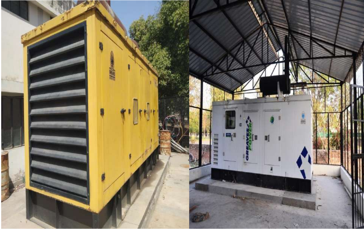
Fig. 3.14: DG Set Installed in Electrical Wing and Estate Office
