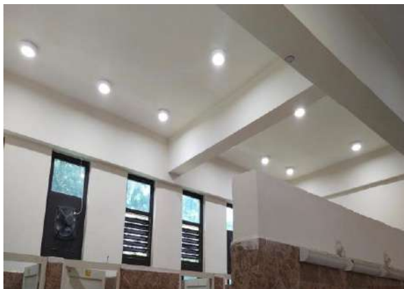
Fig. 3.9: Occupancy Sensor Installed in The Washrooms of Newly Constructed EDP Block
