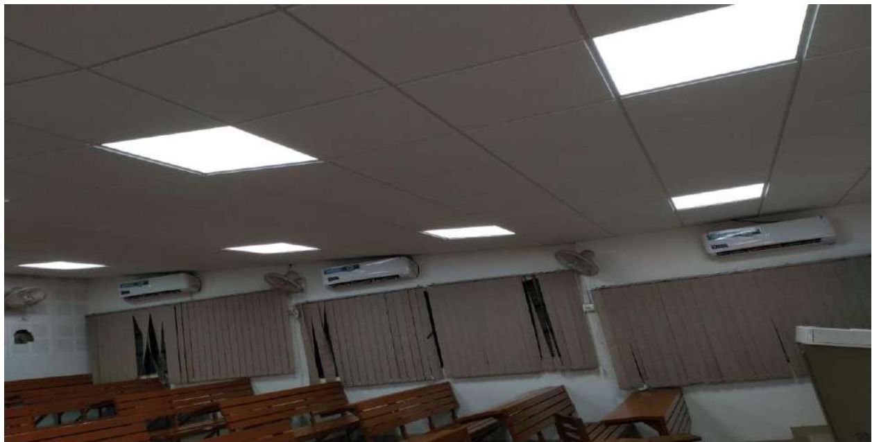
Fig. 3.12: Star Rated Air Conditioning in Smart Classrooms (Food Block, LCF-I)
