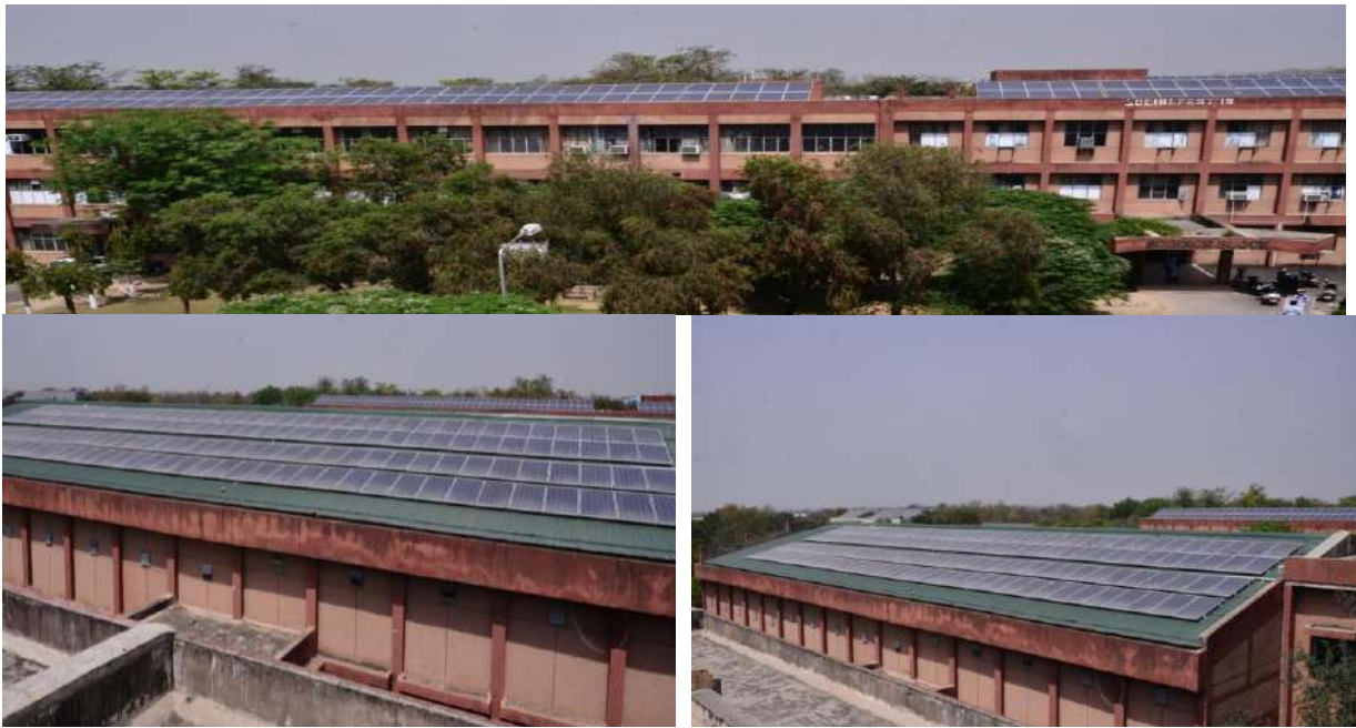
Fig. 3.13: Solar Panel Installed on the Roof Top of Buildings (Science and Mechanical Block)
